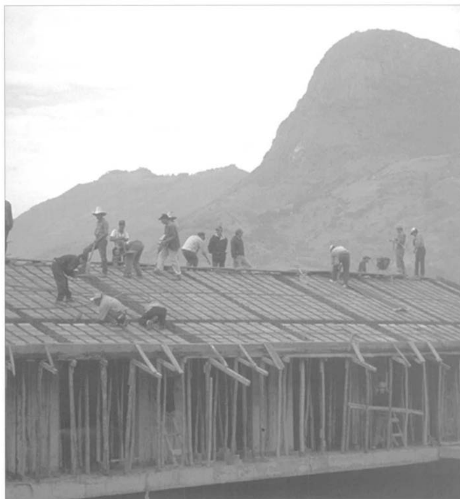
► Government workers on the roof of the new school building in Santo Domingo, Piura
