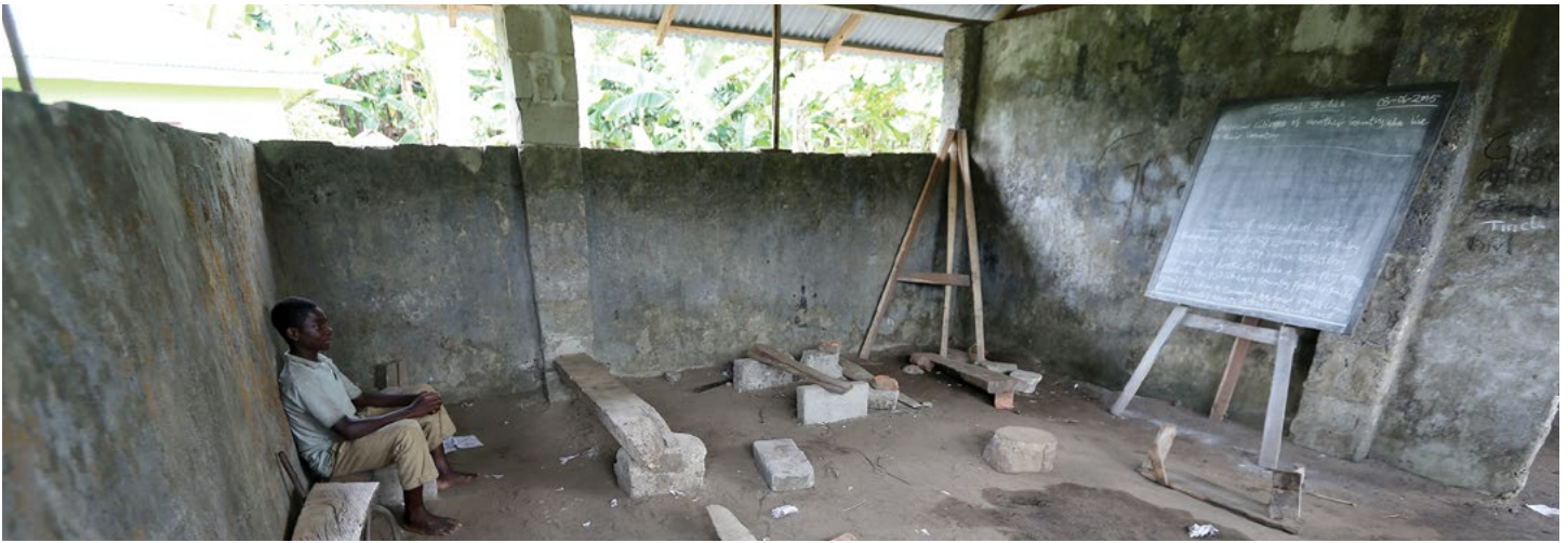
A primary school in Rumuekpe was destroyed in a recent conflict and is now partly rebuilt. Information about oil revenues could help local leaders advocate for more funds for education. George Osodi / Panos for Oxfam America
