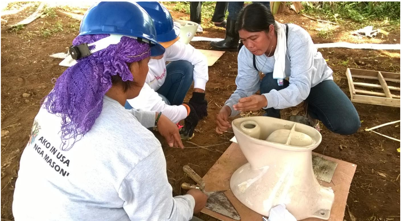
Liezel, a builder from Bantayan Island training more builders in Guiuan, Eastern Samar, August 2016. Photo: Rona Ramos
