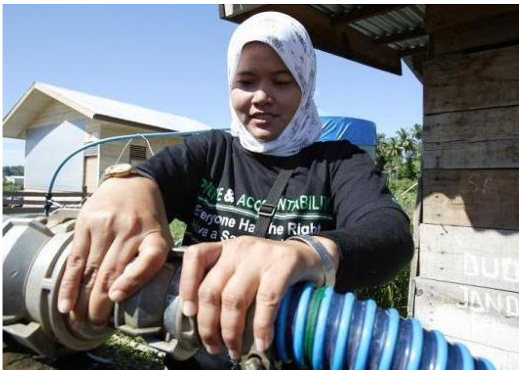
An Oxfam project officer checks a water pipe at the Oxfam pumping station, Aceh, Indonesia (2005). Photo: Jim Holmes/Oxfam
