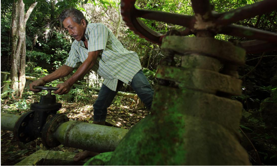
Gravity flow water system installed by Oxfam following by the Indian Ocean tsunami, Lampuuk, Aceh Besar, Aceh Province, Sumatra, Indonesia (2014). Jim Holmes/Oxfam GB
