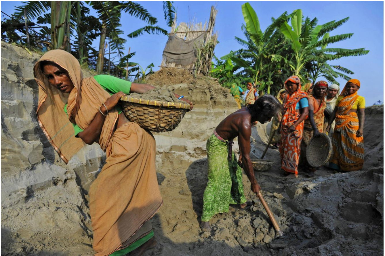
Sufia, with women working as day labourers, help to raise the ground beneath her home to cope with rising seas and high tides, Char Atra, Shariatpur district, Bangladesh (2009). © Dan Chung / Oxfam GB
