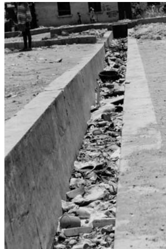
Photo: Example of Solid Waste Blocking Storm Water Drain in Accra, Ghana
