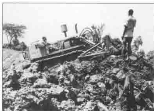
▲ Constructing an earth dam for watering cattle at Toretet, Kericho District – one of the 1960s Oxfam-supported projects in Kenya.
